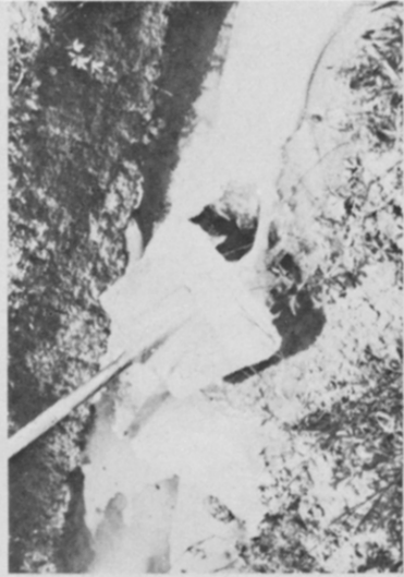
(D) REMOVAL OF GELLED MATERIAL WITH ALUMINUM SHOVEL. MAXIMUM THICKNESS OF CONGEALED CYCLOHEXANE WAS ABOUT 4 INCHES IN THIS EXPERIMENT
